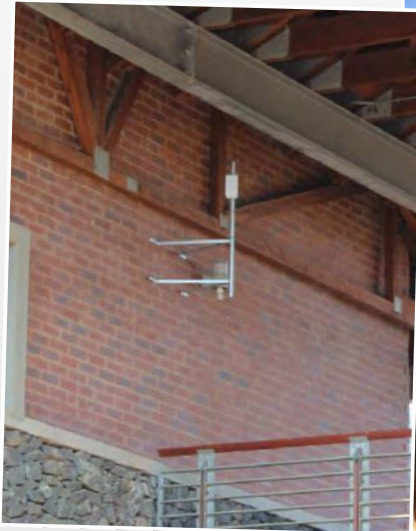
Wireless Transceiver Installation
