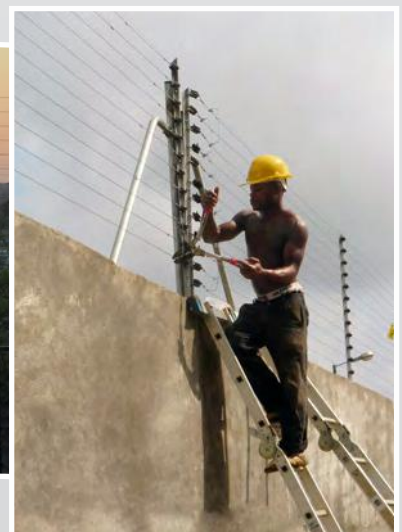
Petro Chemical Plant, Nigeria
