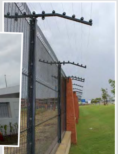
Estate Fence, Midrand (SA)
