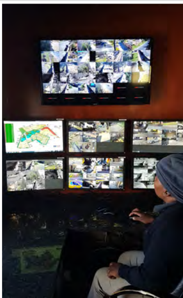
Housing Estate, Control Rooms
