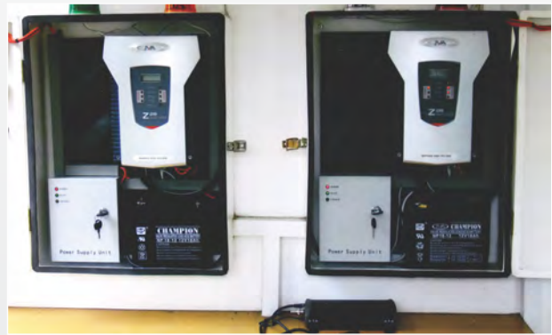
Synchronized System – Internal View
