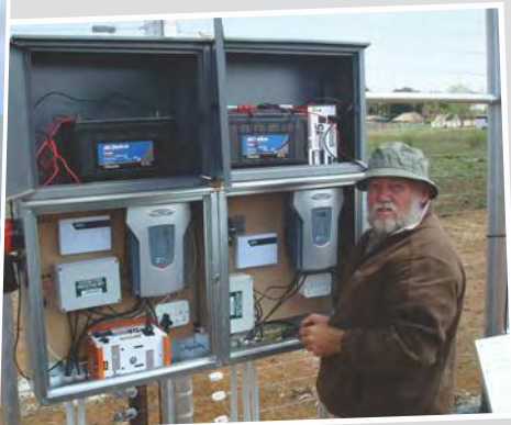
JVA Security Installation, Africa
