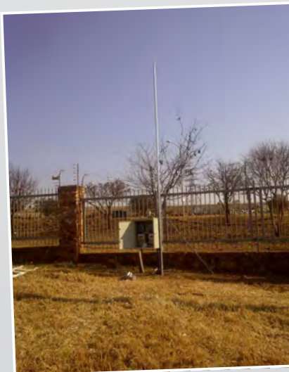
Wireless Repeater Station
