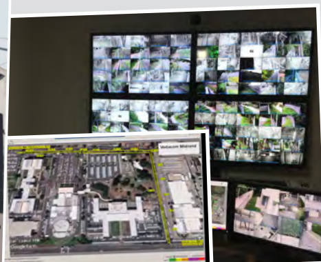
JVA Perimeter Management Systems
