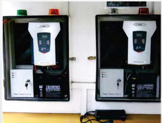
Synchronized System – Internal View
